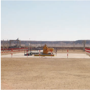
Wellhead, In Salah Gas, Courtesy of BP
